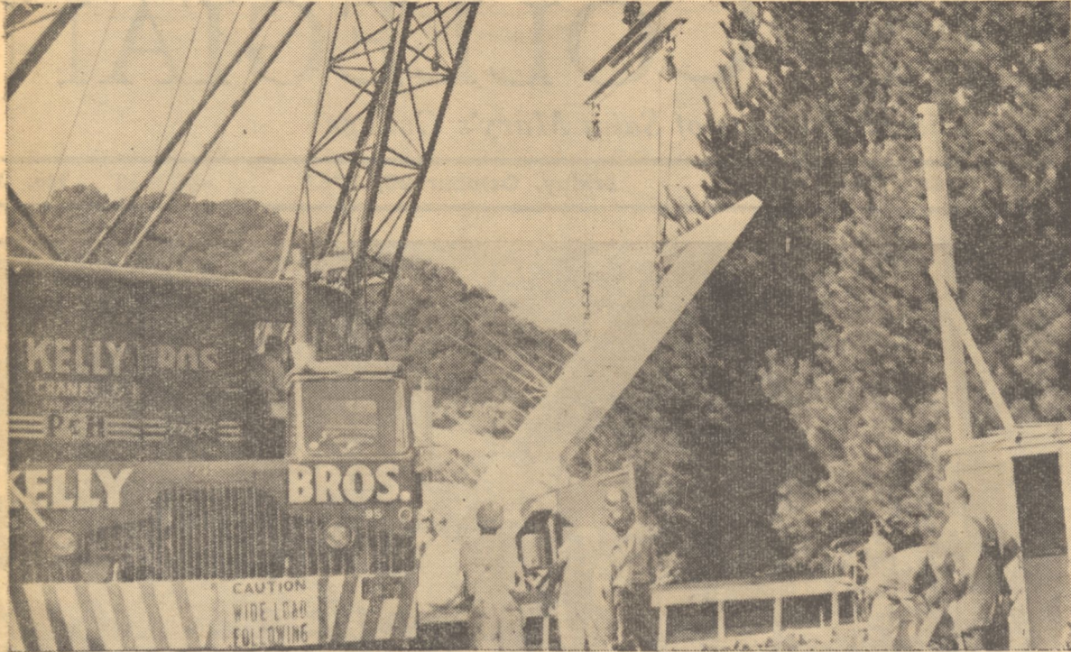
Construction workers shown busily lowering wall in place on construction of new dorms.
