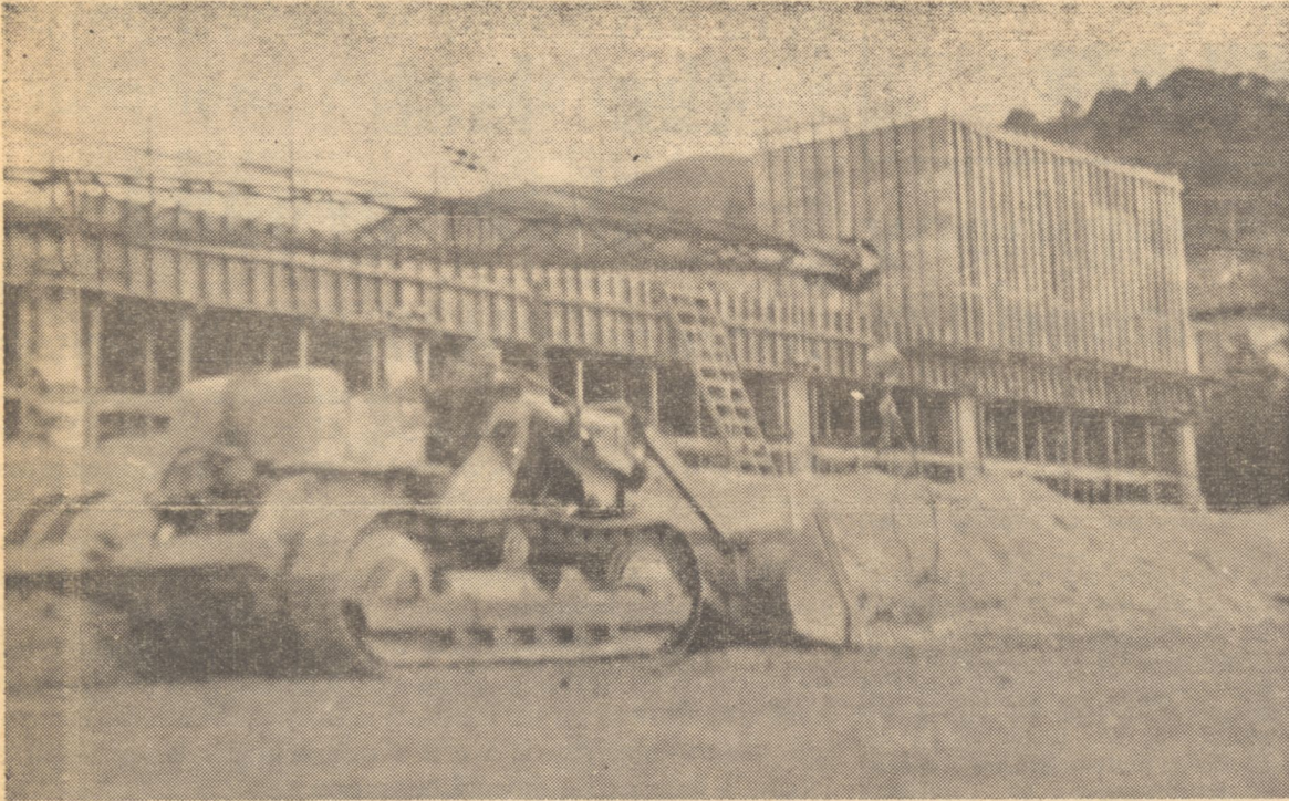
August SAINT ALBERT'S HALL is guarded zealously by tractor and crane. Work on the new library is progressing nearly on schedule, and should be completed in May, according to contracting Barrett Construction Company. The two lower floors have already been finished.
