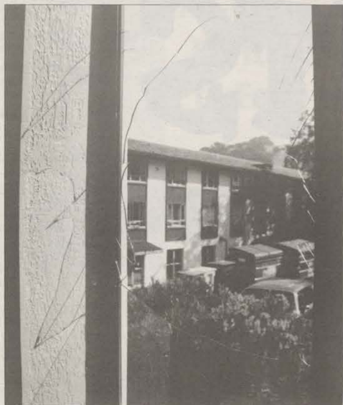
A broken window was found in an Aquinas Hall stairway.
